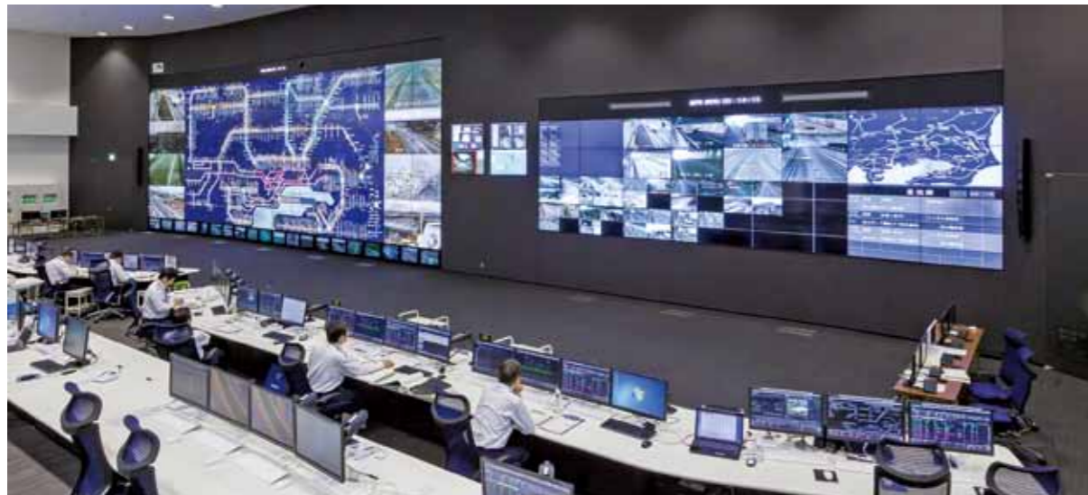
Road Control Center, Kanto Regional Head Office
