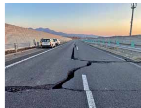
Immediately after the earthquake off the coast of Fukushima Prefecture (Longitudinal and transverse cracks in the paved surface of the Tohoku Expressway)
