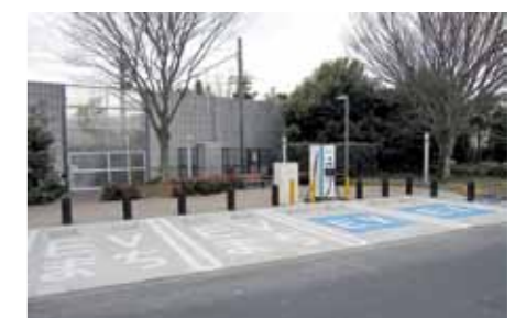
EV quick-charging stations (Keiyo Expwy. Makuhari PA (Inbound))
