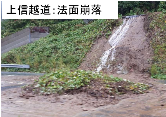
圏央道:法面崩落
