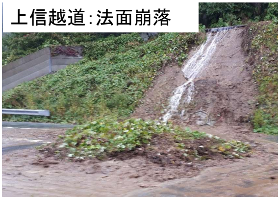
圏央道:法面崩落
